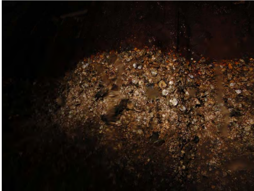
Photo 1: Typical Heavy Marine Growth on Sheet Piling from the Mudline up to the Tidal Zone.
