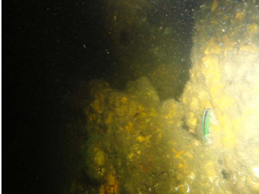
Photo 5: Larger Hole Through Sheet Piling Extending into Concrete Face of Caisson. This hole is located near the west corner of the South face of the Northwest Building Caisson.
